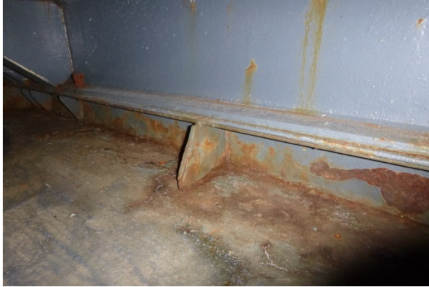
Figure 8: No. 2 Engine Foundation
